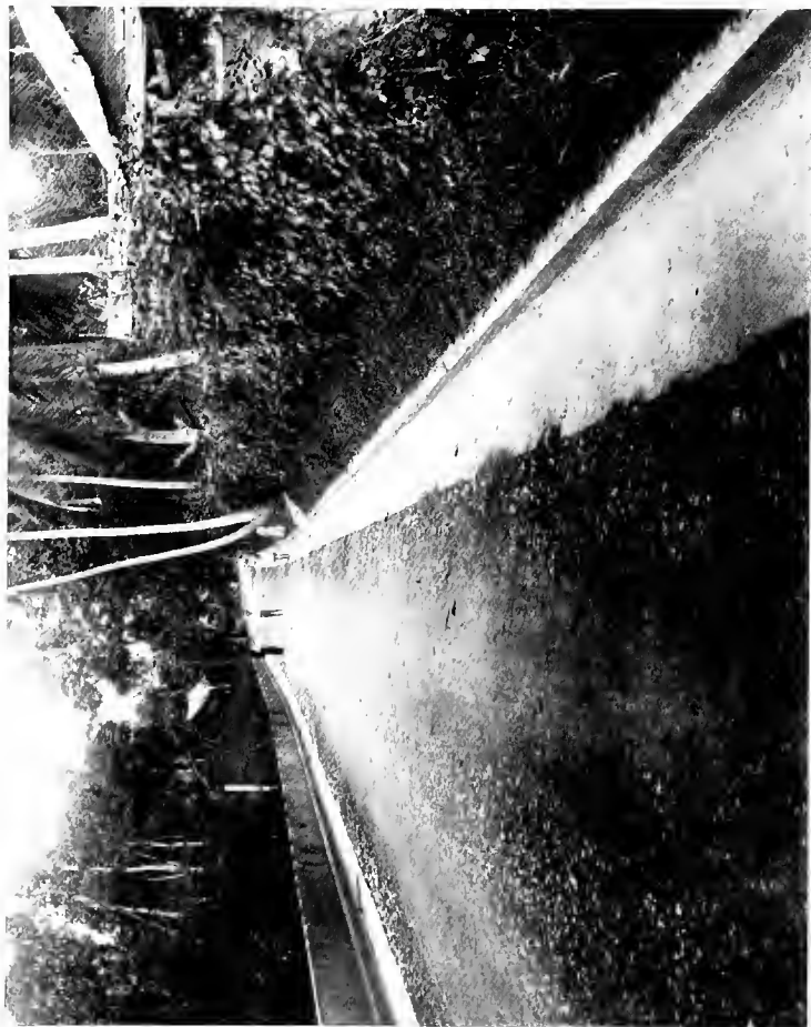
FIG. 24.—A ROAD IN PORT OF SPAIN, PROPERLY GRADED WITH WELL-MADE CONCRETE SIDE DRAINS.
